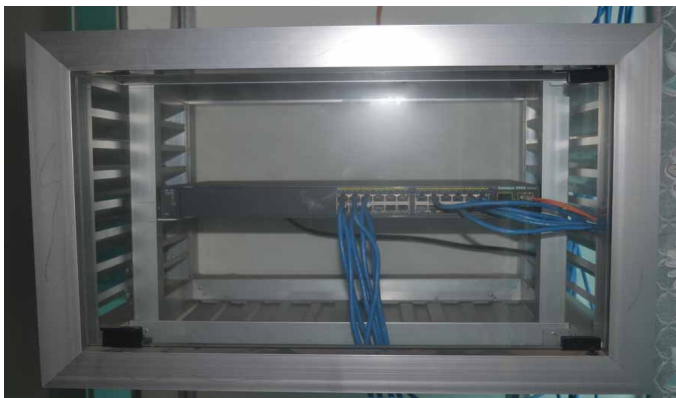
A sample image for an existing switch rack.
