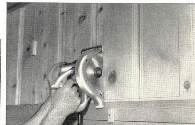
↑ Entering panelled wall with a pocket cut in preparation for a built-in cabinet.
